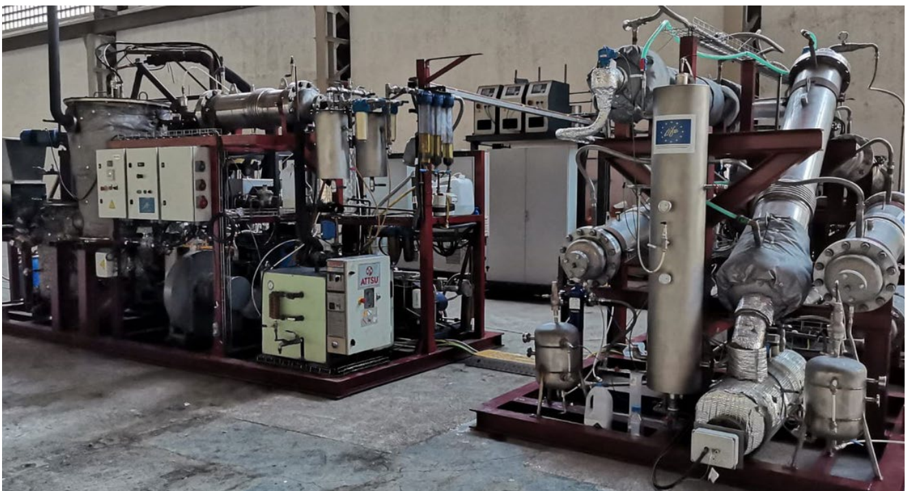
BluePlasma Power's Gasification Plant
