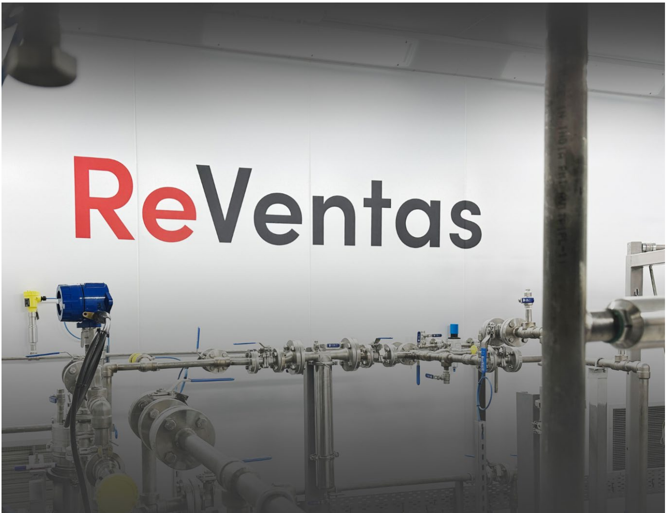
ReVentas technology pilot plant
